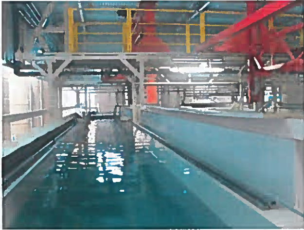
Polypropylene pretreatment tanks
