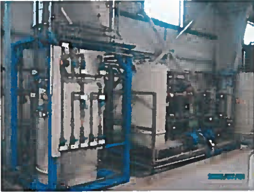
UF plant (paint recycling)
